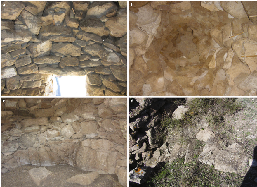
Fig. 5. Constructive details: (a) relieving arch above the entrance, (b) inner part of the roof, (c) direct contact of the basement to the rock, (d) stone ramp.
