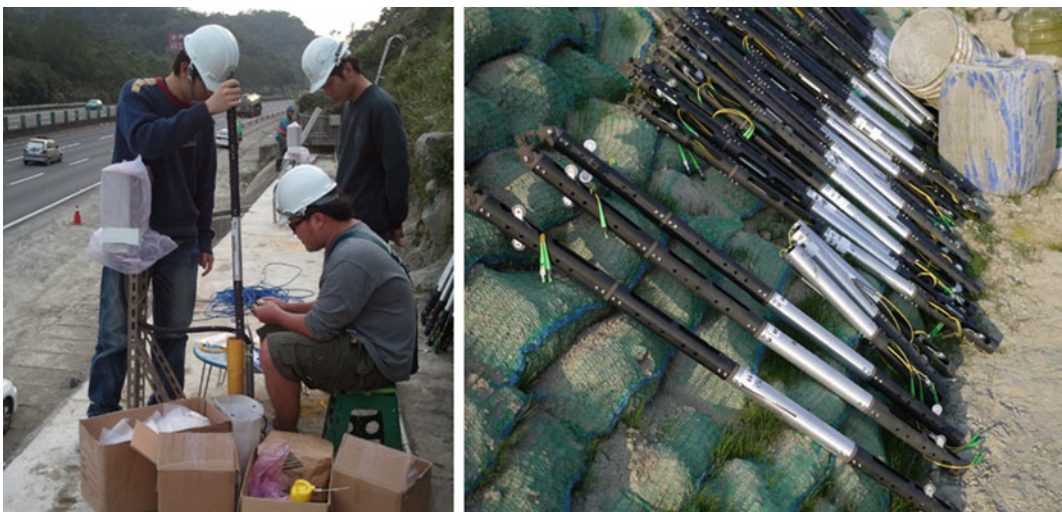
Fig. 13 The fibre optic Bragg grating (FBG) in-place inclinometer
