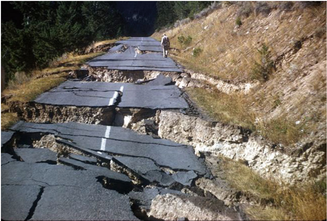
Fig. 18 Lateral spreads at Hebgen Lake near West Yellowstone, Montana (USA), due to the effects of the Magnitude 7.3 Hebgen Lake earthquake, on August 18, 1959. Photo by R.B. Colton, U.S. Geological Survey
