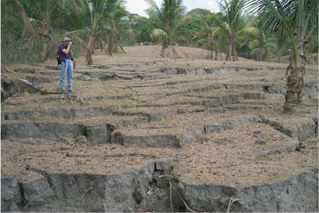
Fig. 20 Lateral spreading caused by the magnitude 6.5 El Salvador, Central America earthquake of February 13, 2001. Area shown is on the eastern shore of Lago de Ilopango. Photograph by Anthony Crone, U.S. Geological Survey
