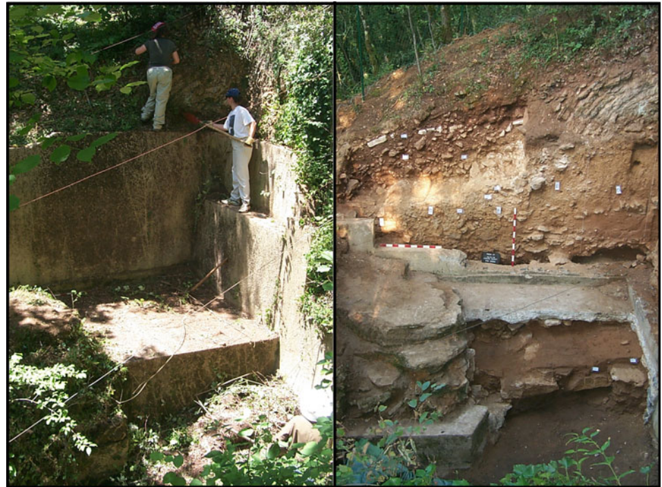
Fig. 1.14 ( left ) Pech IV looking west prior to the demolition of the cement wall and ( right ) after partial removal of the wall. For reference, the flat bench on the left is the same as the flat bench still partially intact on the right
