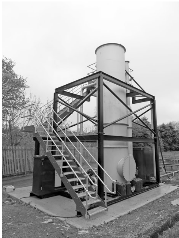
Fig. 26.5 Full-scale, expanded bed biofilm reactor (EBBR) prototype package plant (Technology Readiness Level 7) constructed in stainless steel by J. K. Fabrications, Newry, Northern Ireland. The expanded bed column is 1.5 m diameter and the expanded bed depth is 5 m. This size of EBBR is able to nitrify at least 8.8 kg \text{NH}_3\text{-N} per day, which is equivalent to purifying the secondary effluent from a population of about 2200 people
