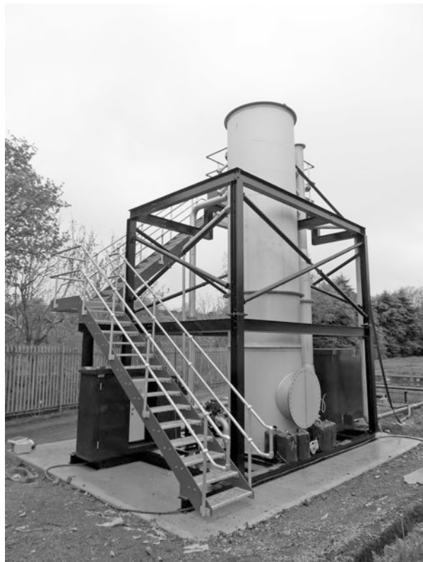
Fig. 26.5 Full-scale, expanded bed biofilm reactor (EBBR) prototype package plant (Technology Readiness Level 7) constructed in stainless steel by J. K. Fabrications, Newry, Northern Ireland. The expanded bed column is 1.5 m diameter and the expanded bed depth is 5 m. This size of EBBR is able to nitrify at least 8.8 kg \text{NH}_3\text{-N} per day, which is equivalent to purifying the secondary effluent from a population of about 2200 people
