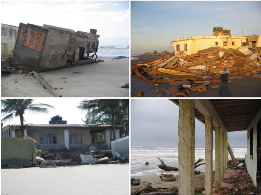
Fig. 24.3 Houses destroyed by coastal erosion in Ponta Norte of Ilha Comprida (2014). Source Roberto Frozza 2014
