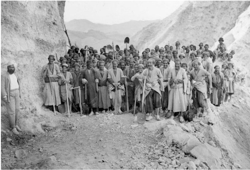
Fig. 3 Construction of the Gach-qaraguli (Gachsaran) Road, 1909. Source British Petroleum Archive, Warwick, Britain.
