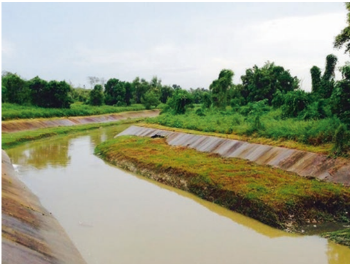
Fig. 4.18 Sediments is accumulated on the concrete river and colonizing the manmade river (Photo taken by authors 2016)
