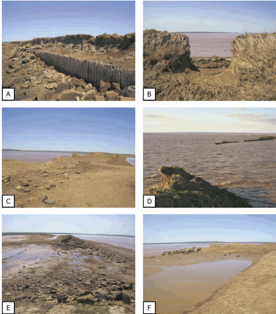
Fig. 21.16 Photographs illustrating erosion of the old dike from October 2012. Panels a–f are described in the accompanying text (Photographs by Jeff Ollerhead)
