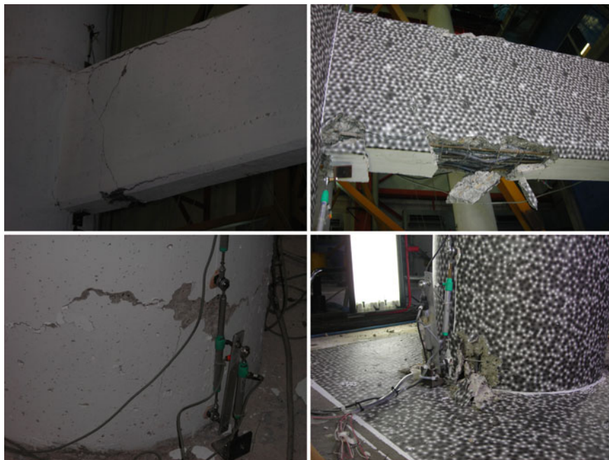
Fig. 6.8 Crack pattern in the transverse beam ( top left ) and base column ( bottom left ) of the tall pier and buckling of the transverse beam ( top right ) and base column ( bottom right ) after k12 test (PGA = 200% ULS)
