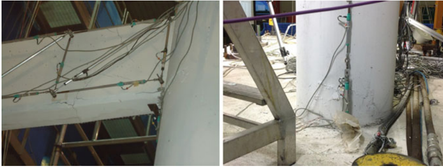
Fig. 6.7 Shear cracks pattern in the transverse beam ( left ) an column ( right ) of pier 11 after the test k09 (ULS PGA = 100%)
