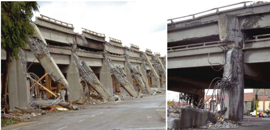
Fig. 6.1 Typical damage experienced by existing reinforced concrete bridges after an earthquake: sliding shear at top columns of the Cypress viaduct in the 1989 Loma Prieta earthquake (after NISEE, 2000)
