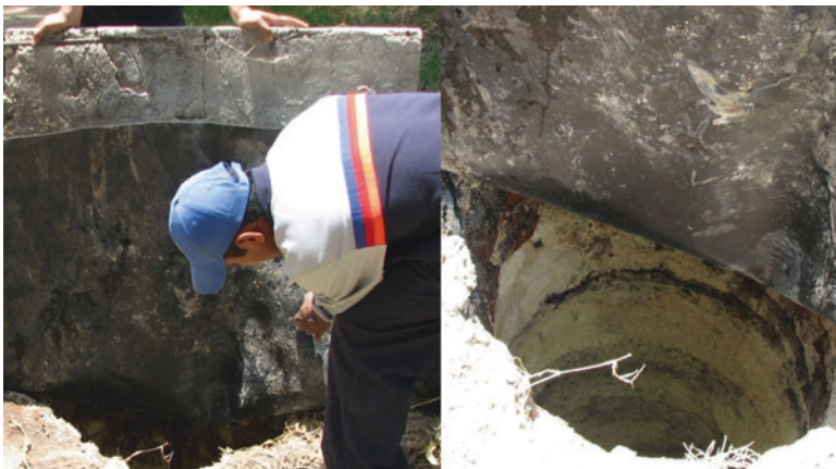
Fig. 2.3 Sulfur deposits at the visiting manholes of experimental site
