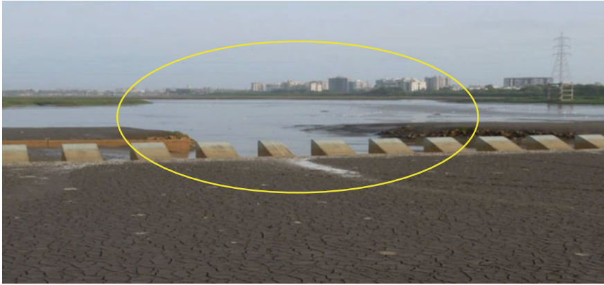
Photo 1 Damaged portion of the first span (Ch. 40–310 m) at downstream of Singapore weir, Surat
