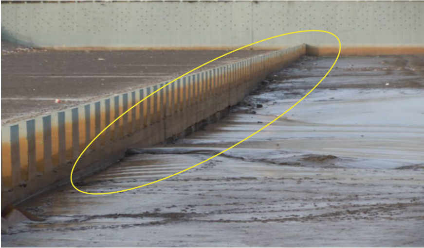
Photo 2 Displacement of concrete blocks from its mean position of the first span (Ch. 40–310 m) at downstream of Singanpore weir, Surat
