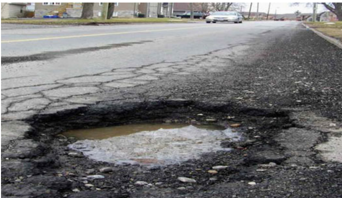
Fig. 4 Another pothole in Bengaluru
