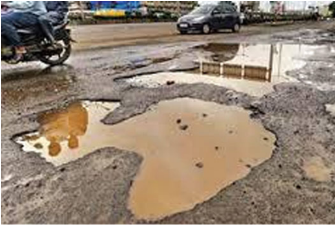
Fig. 3 Pothole in Bengaluru
