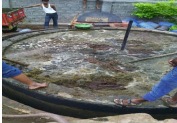
Fig. 1 Observed scum in the baseline digester
