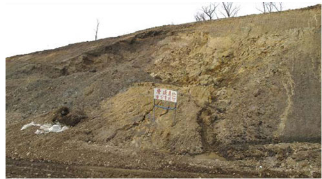
Fig. 10 Landslide on the cut slope (2012.4.23)
