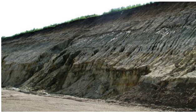
Fig. 4 Groundwater out flowed and eroded the cutting slope
