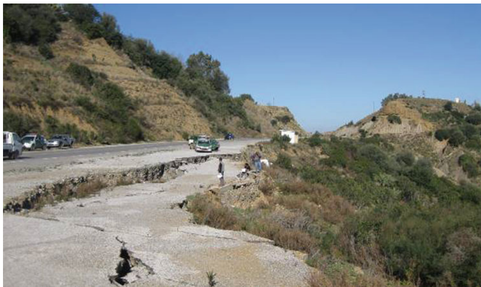
Fig. 5 Landslide occurred along the national road RN77 in Miocene marine formation (weathering profile)
