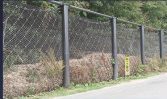
SLOPE GUARD FENCE: Slope failure protection fence caught soil of slope failure caused by a heavy rain.
