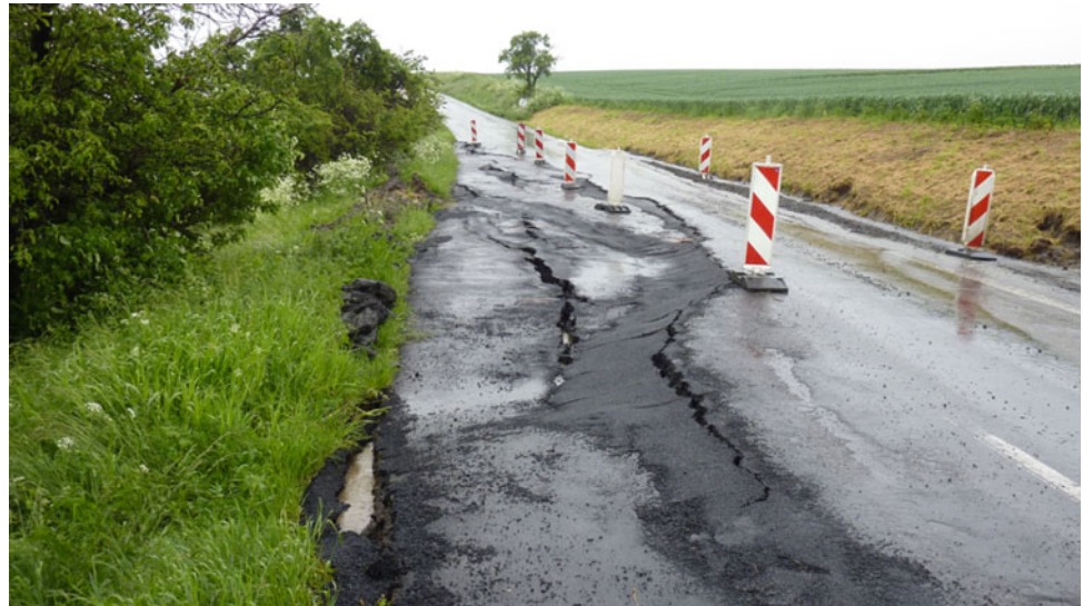
Fig. 8 Road II/432 between Koryčany and Jestřabice in the Zlín region destroyed by a landslide in May 2010. Cracks were up to 15 cm wide and tens of cm deep. Photo: Michal Bíl, May 2010
