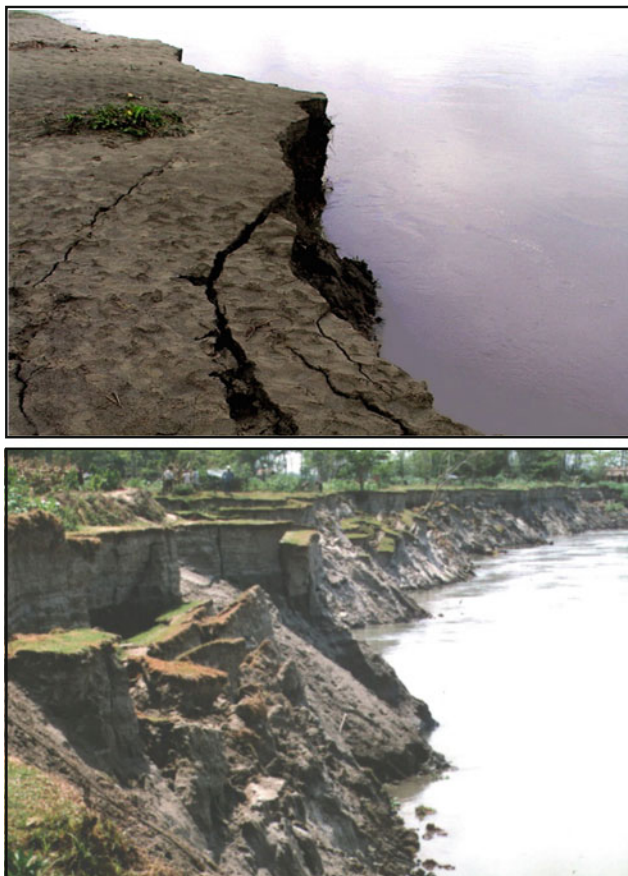
Fig. 3 Bank Erosion in the Brahmaputra River
