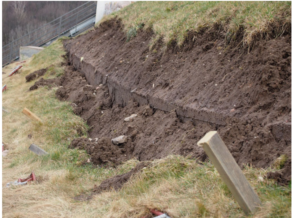
Fig. 6 Retaining pile caps exposed in February of 2016 by formation of shallow landslide of frontal type (photo by Vidas Mikulėnas)
