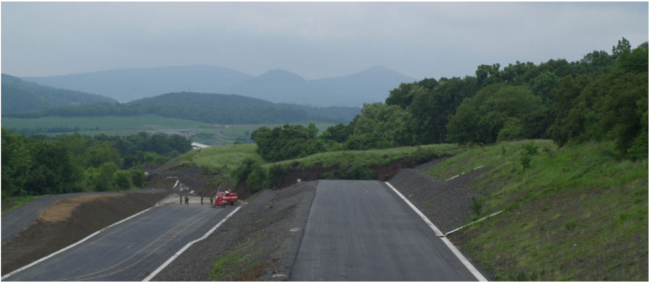
Fig. 1 An example of an extremely devastating landslide which destroyed D8 motorway in June 2013. The motorway was under construction at the time of the event. The direct losses, including the
