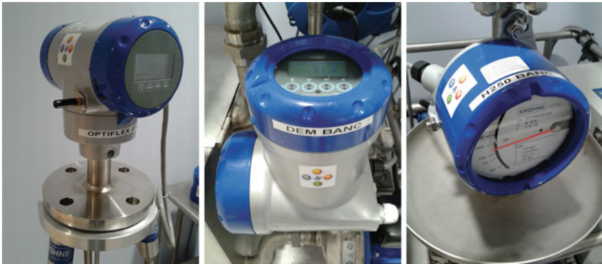
Fig. 22 Examples of sensors for process monitoring using the OCARI protocol
