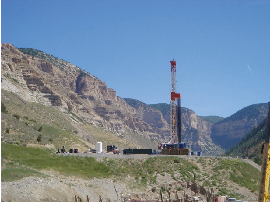
Fig. 4.10 Remote natural gas well. Source: https://www.flickr.com/photos/25069384@N03/8743405319 , 2016
