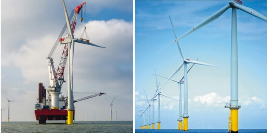
Fig. 6.5 A part of London Array containing 175 Siemens 3.6 MW wind turbines (rotor diameter 120 m, hub height 87 m), floating crane is used for installation of blades (on the left side ). Source: London Array Limited: How a turbine works, 2016, http://www.londonarray.com/how-a-turbine-works/
