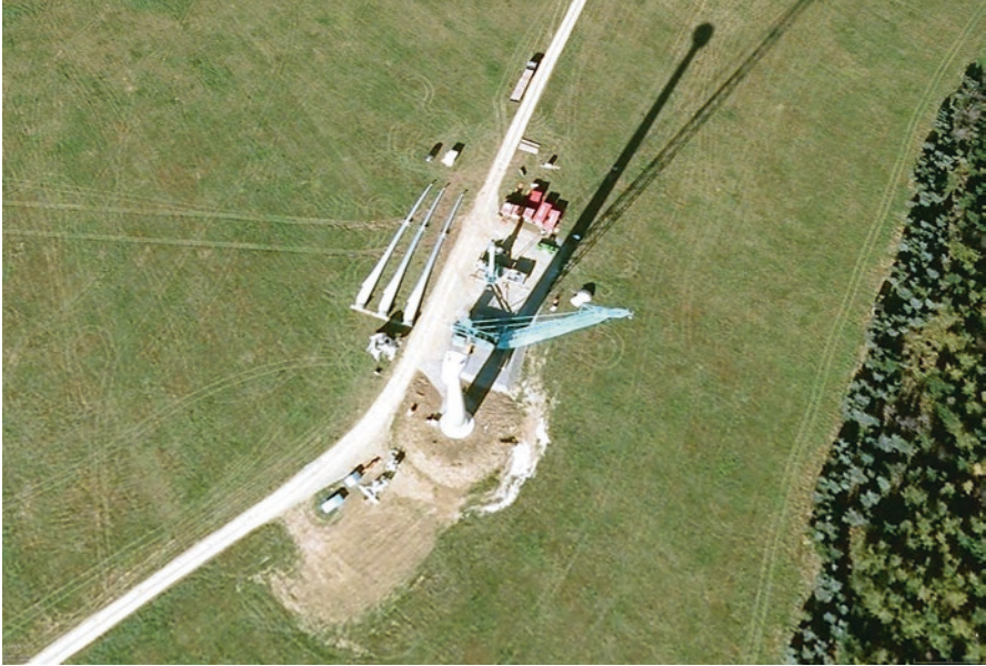
Fig. 6.22 A detailed view on the installation of a wind turbine (2 MW). Google Earth, 2016
