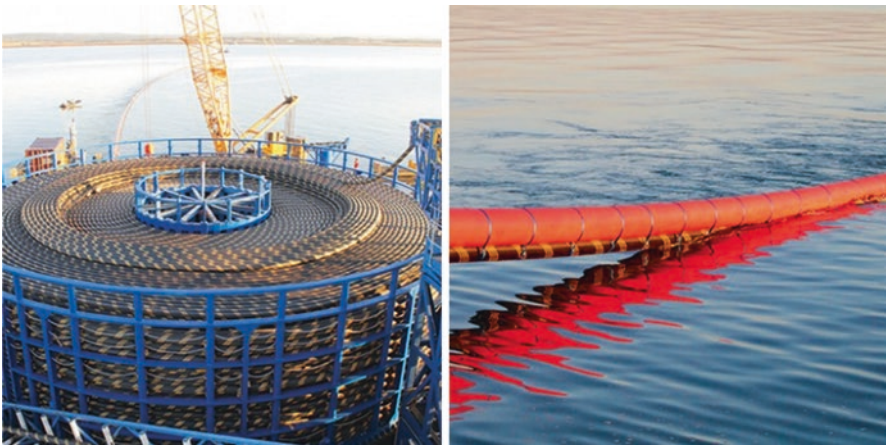
Fig. 6.6 An example of connection to the electrical grid and its installation (on the left side ). Source: London Array Limited: How a turbine works, 2016, http://www.londonarray.com/how-a-turbine-works/
