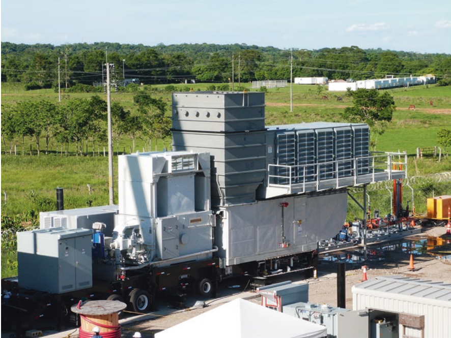
Fig. 4.11 Mobile gas turbine used to generate electricity. Source: www.pixabay.com
