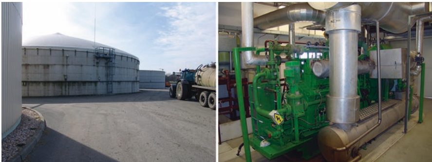
Fig. 8.4 Devices of a biogas power plant: the anaerobic digesters and the power generator (on the right side )
