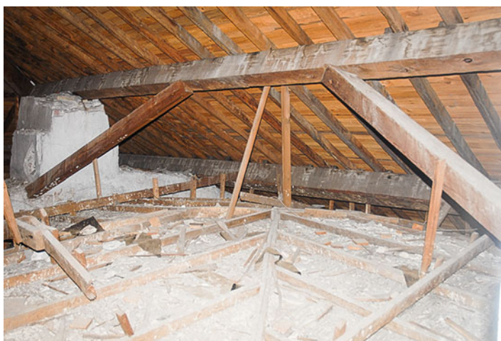
Fig. 6.34 Flat frame system in the northern tower: the horizontal purlins rest on a spine wall and on pillars built over large masonry arches; their span is reduced through the insertion of braces. Below the roof, we have an example of a hanging wattle vault
