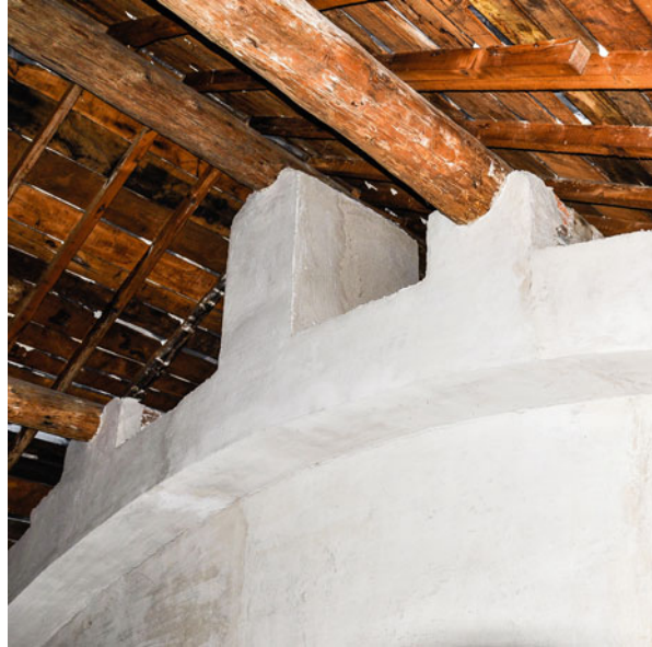
Fig. 6.24 Primary beams supported by short pillars on arches in the coverings of the northern wing of the central cross (CN)
