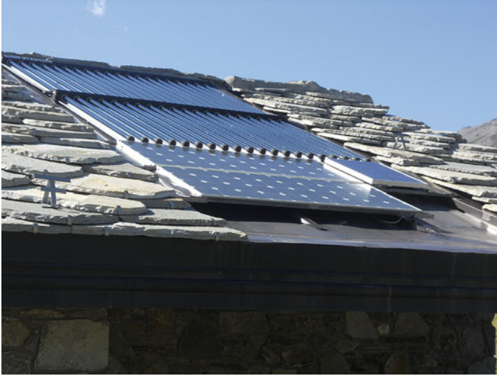
Fig. 9.7 Alpine roof, Italy. Caotic attachment of solar and PV panels
