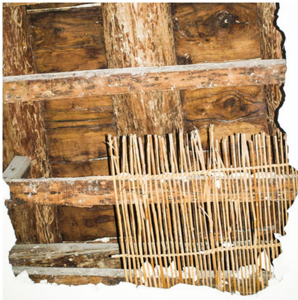
Fig. 6.16 False ceiling of a flight of stairs: the reed mat is bolted to a series of common rafters fastened at the soffit of the flooring system elements
