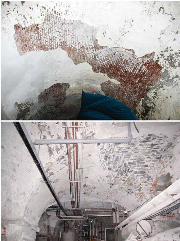
Fig. 6.8 Examples of vaults on the bottom floors: barrel vaults in bricks and groin vaults in stone
