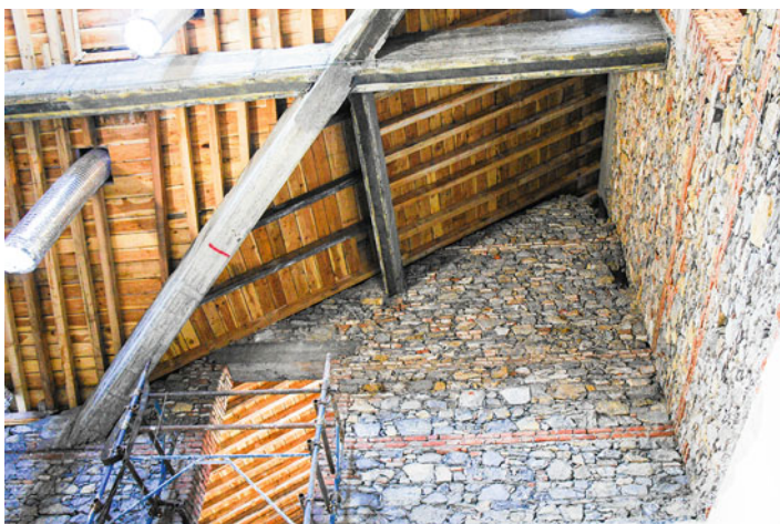
Fig. 6.6 Post-war reconstruction of masonry works in the advanced central body. We may observe the insertion of horizontal brick courses in the masonry characterized by irregularly shaped stone elements
