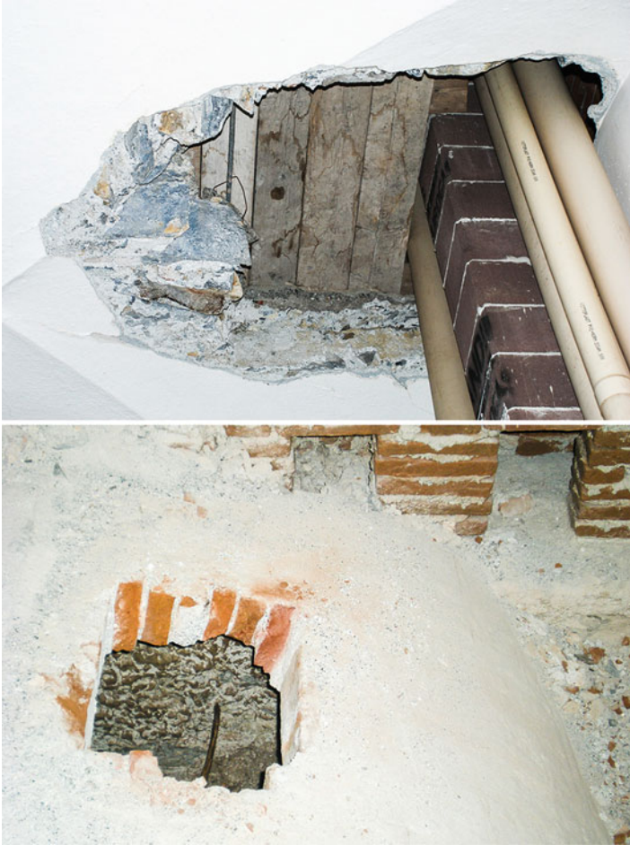
Fig. 6.9 Groin vault in hewn stone (at the top ). Brick vaults have in the wrench a minimum thickness of one head (at the bottom )
