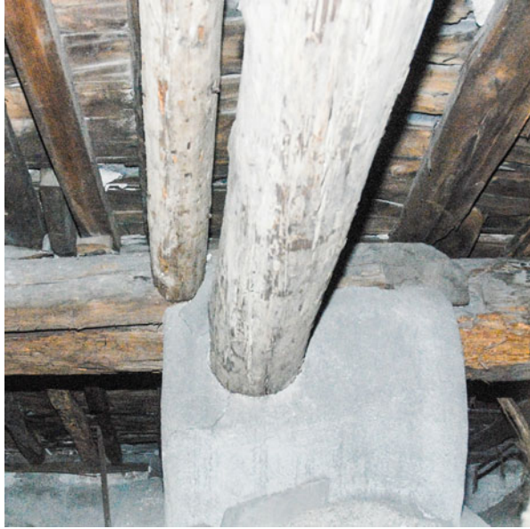
Fig. 6.27 On the small pillars rest the horizontal purlins and the struts sustaining the next order
