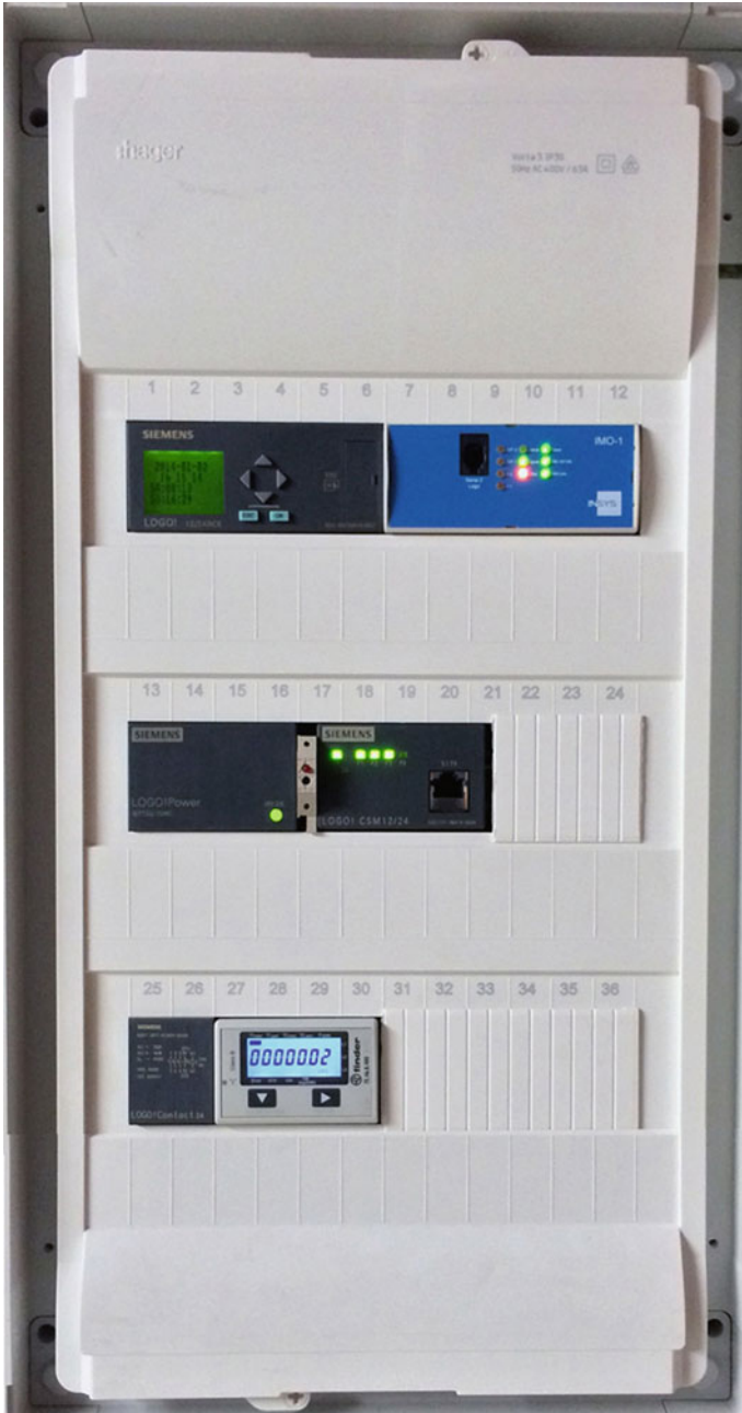
Fig. 3 Center of stationary assistance subsystem with Siemens LOGO™ SPS/PLC and insys IMO-1™ rule-based fault transmitter and GPRS router ( upper row ), power supply, industry IP switch ( middle row ) and electric power sensor and contactor for the electric stove ( lower row ) in a standard 3-row junction box
