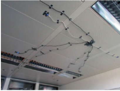
(a) The layout shows the six EPIC sensors placed on the ceiling to cover the test room [3]
