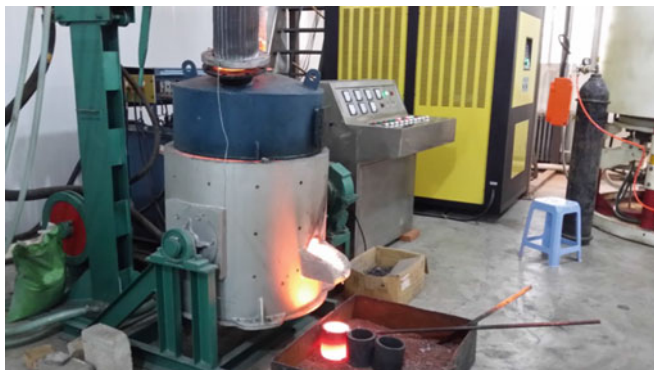
Fig. 1 100 kVA DC submerged arc furnace
