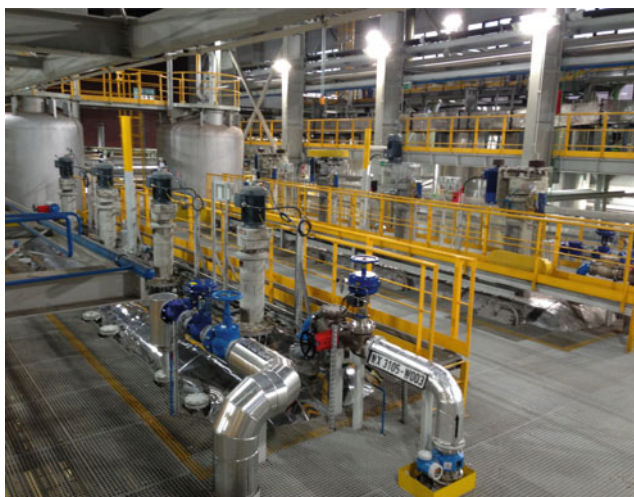
Fig. 2 Waelzoxide treatment plant at ZGH Bolesław S.A.—pressure washing
