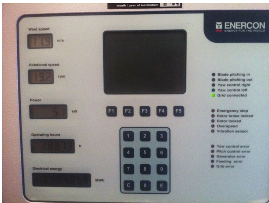
Fig. 4.11 Digital display and control panel in Tilley (photograph © William Simm)
