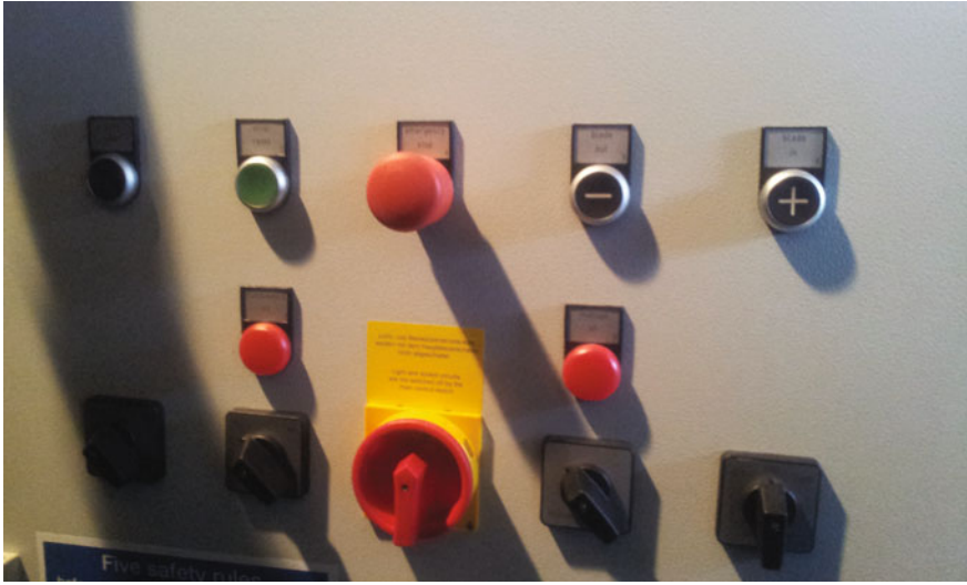
Fig. 4.12 Physical control panel in Tilley (photograph © Maria Angela Ferrario)
