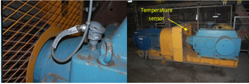
Fig. 1 Conveyor belt gearbox and the temperature sensor
