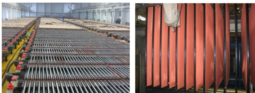
Fig. 8 Tankhouse with METTOP-BRX Technology at Xiangguang Copper ( left ) and excellent surface quality of the cathodes
