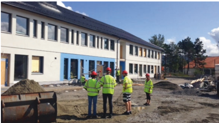
Fig. 13.2 This photo shows inmates and employees in front of the new prison building under construction, discussing details and outlines of the building
