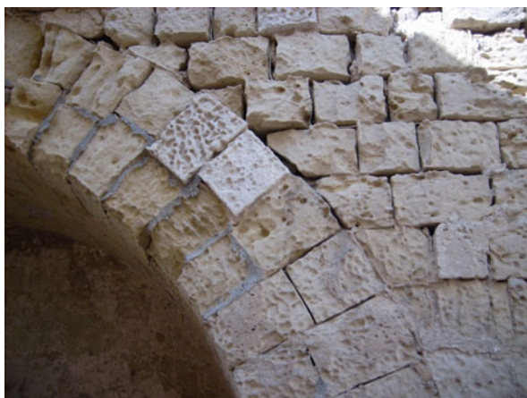
Fig. 3.13 Historical center of La Valletta: calcarenite blocks affected by alveolarization
