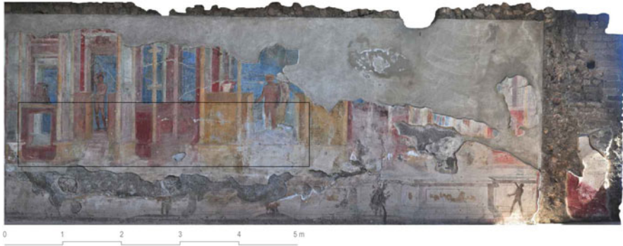
Fig. 29.13 The Gymnasium: Orthophotograph of the south wall painting. The black rectangular box denotes the area of fresco investigated by GPR
