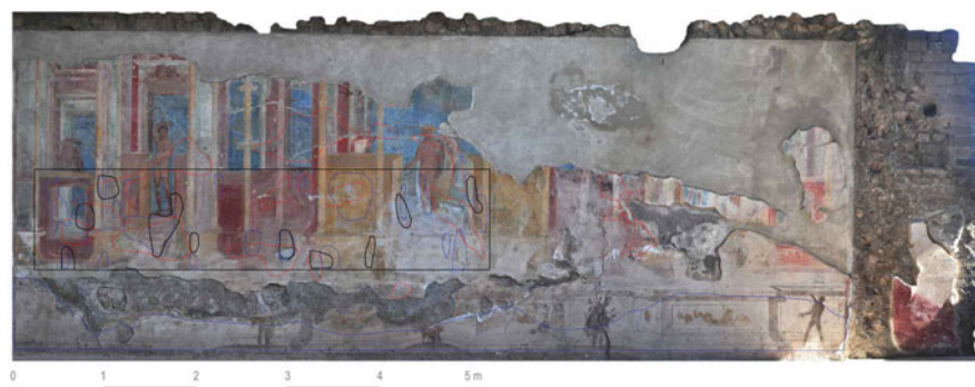
Fig. 29.17 The Gymnasium: Detail of the wall painting. Black and light blue lines border areas characterized by high-amplitude GPR at 3.5 and 4.7 cm depth, respectively. Red lines border areas characterized by thermal anomalies. Blue lines indicate areas affected by rising. The images show that most of the thermal anomalies are characterized by GPR at high amplitude at 3.5-cm depth, likely resulting from the presence of detachment or scarce adherence between the plaster layers of the fresco
