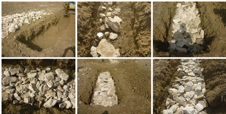
Fig. 7.4 Photographs taken during the construction of the test field in Alampra village, in central Cyprus (Photograph by A. Agapiou)
