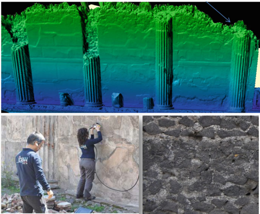
Fig. 29.2 Top : Digital model of southern wall of the Basilica investigated by GPR and seismic tomography. The wall is interrupted by plastered fluted semicolumns built with bricks. Bottom left : GPR data acquisition. Bottom right : Detail of the masonry composed of irregular stone elements of Peperino
