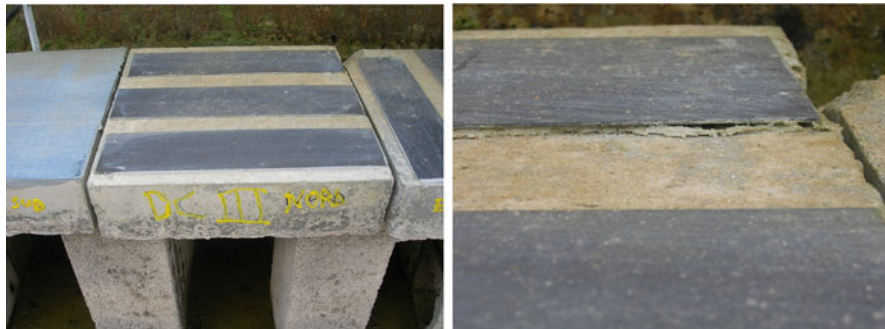
Fig. 11.12 View of realized specimen on site ( Left panel ) – Detailed view at plate level
