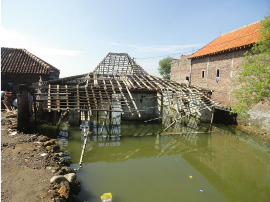
Fig. 8.5 Three stages of unsustainable adaptation of type 1 housing in an inundated Bedono Village. From left to right, 2nd stage development, 1st stage inundation, 3rd stage development (Source private collection 2013)
