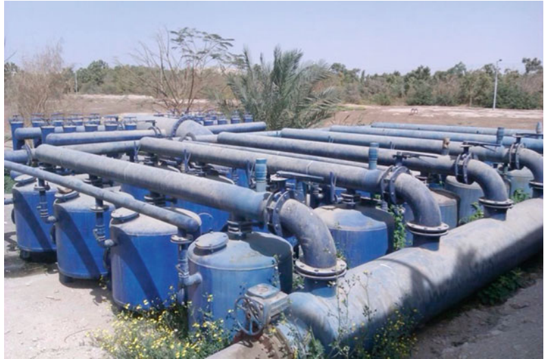
Fig. 14.7 Sand filters for the crude wastewater
