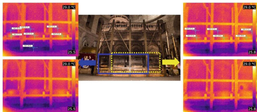
Fig. 9.10 IR-thermal inspection of the south façade of the Holy Aedicule of the Church of the Holy Sepulchre
