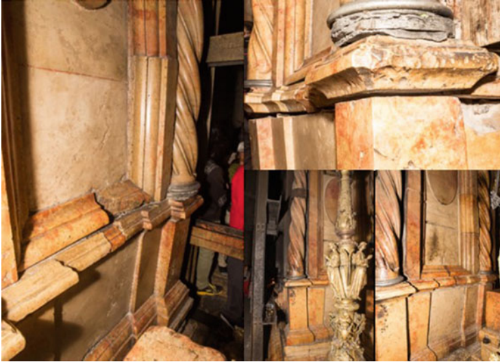
Fig. 9.8 External facades deformations
