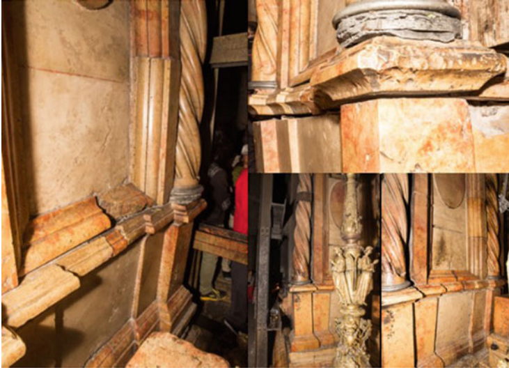
Fig. 9.8 External facades deformations
