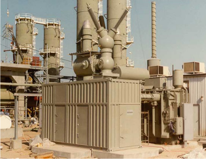
Fig. 16.4 First containerized substation 145 kV in 1985 with machine transformer
