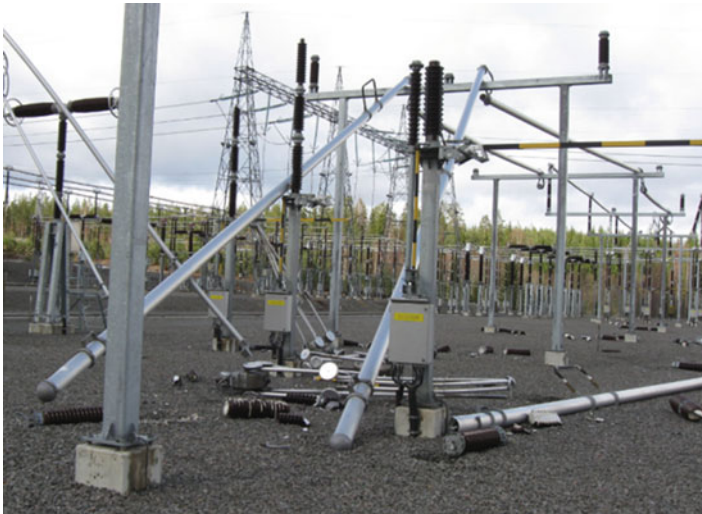
Fig. 12.24 Collapsed 400 kV busbar caused by vibration
