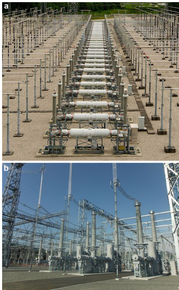
Fig. 16.3 (a) 420 kV hybrid installation with GIS and air-insulated busbar. (b) 550 kV hybrid installation with GIS and air-insulated busbar
