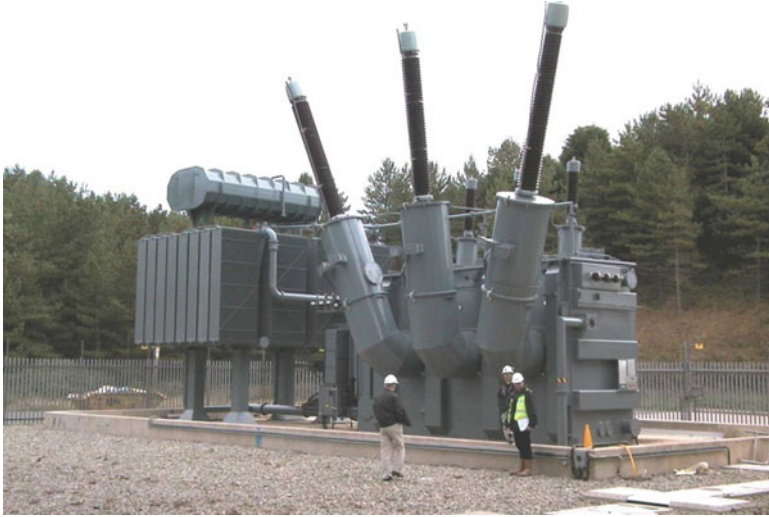
Fig. 12.46 Typical 400/132 kV transformer
