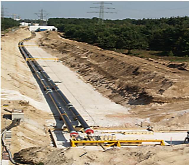
Fig. 27.15 Overview of directly buried GIL at Kelsterbach, Germany, 2010
