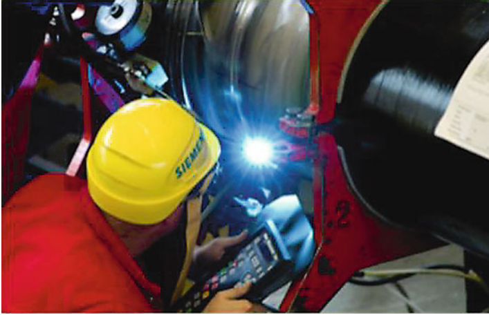
Fig. 27.28 Orbital welding machine for enclosures and phases
