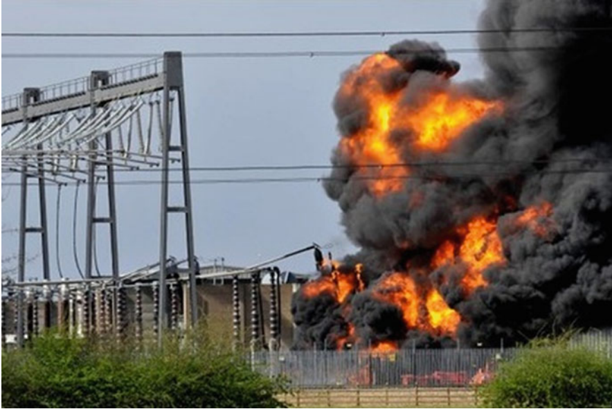
Fig. 5.12 A transformer fire in a 400 kV substation
