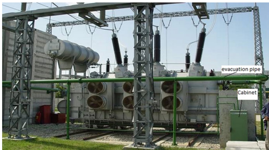
Fig. 11.35 Transformer fire suppression using nitrogen in Romania
