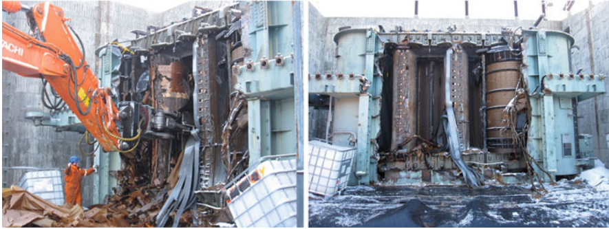
Fig. 45.1 Left: ongoing breaking up of a 170 MVA, 220/110 kV transformer in the substation. Right: the site when the work with two phases is complete
