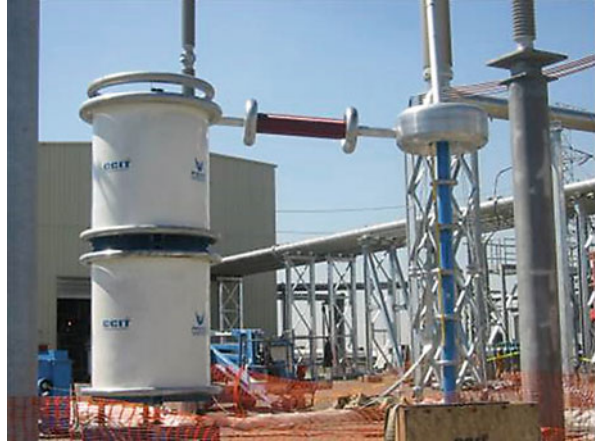
Fig. 27.36 On-site HV testing air insulated high-voltage resonance test setup connecting to the bushing
