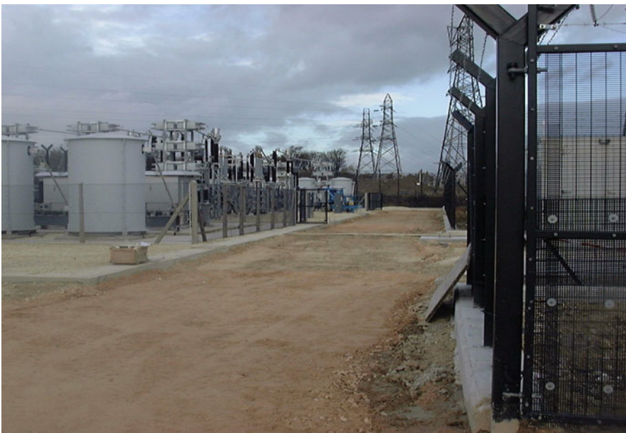
Fig. 5.14 External fence around a substation with the same level of security as a prison
