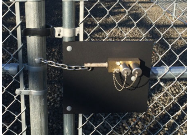
Fig. 14.8 Example of key interlocking system
