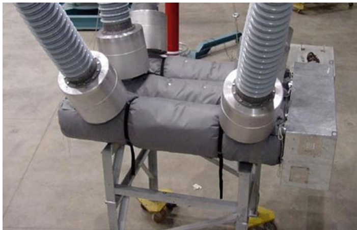
Fig. 12.55 Jacket or blanket heating on circuit breaker
