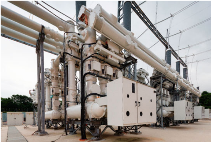
Fig. 15.1 420 kV GIS with overhead line
