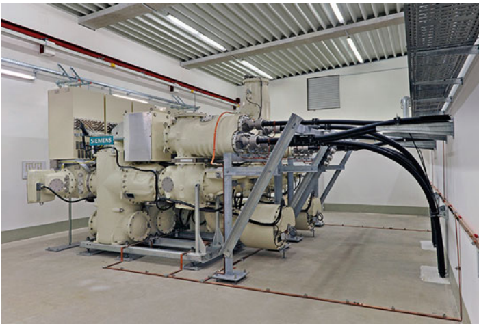
Fig. 15.2 145 kV GIS with cable connection
