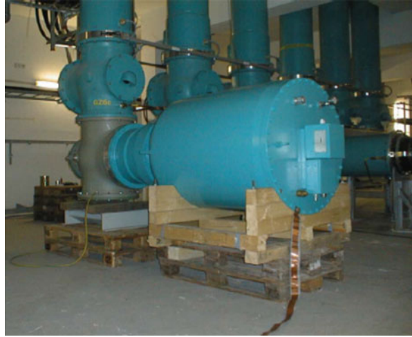
Fig. 27.34 Gas insulated high-voltage resonance test set-up. Max. voltage 680 kV, max. current 1,5 A, L = 720 mH
