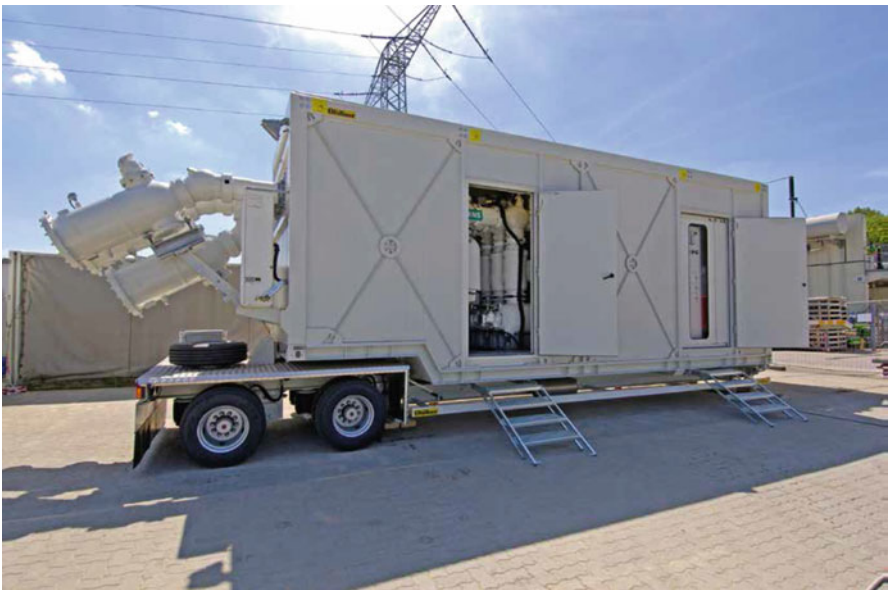
Fig. 6.4 Mobile substation next to main substation
