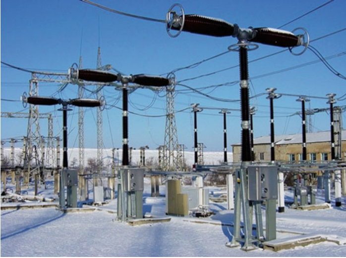
Fig. 12.2 Live tank circuit breakers
