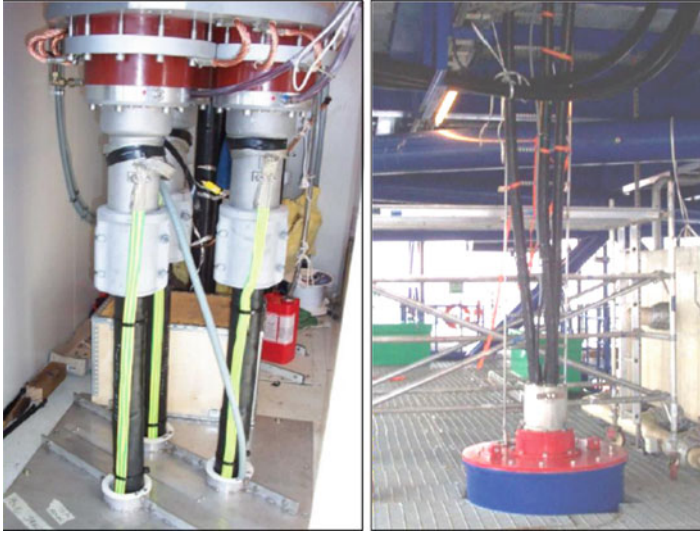
Fig. 29.20 Hang-off block anchoring a high-voltage three-core cable (right) and entry for a connection to a GIS substation
