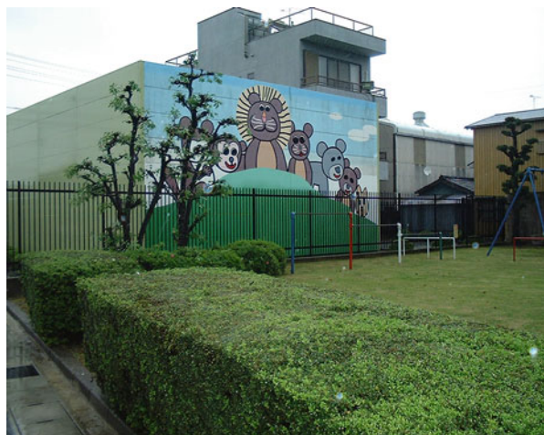
Fig. 42.1 An invisible substation designed for an urban environment adjacent a playground in Japan (Biewendt et al. 2002)
