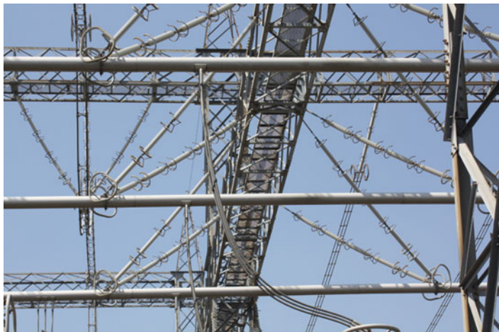
Fig. 12.34 Underhung multiple “long rod” insulators supporting busbars for additional earthquake resilience
