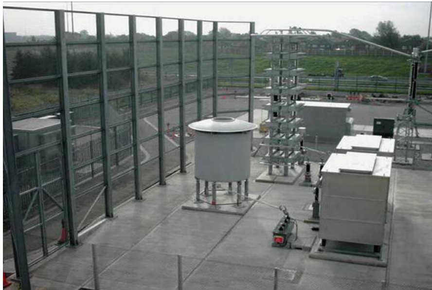
Fig. 11.49 Example of stone guard fencing to protect capacitor banks against vandalism
