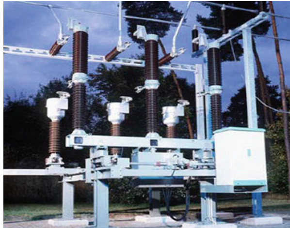
Fig. 26.6 Switchgear with compact bays and conventional components (CIGRE Brochure No. 390 2009)
