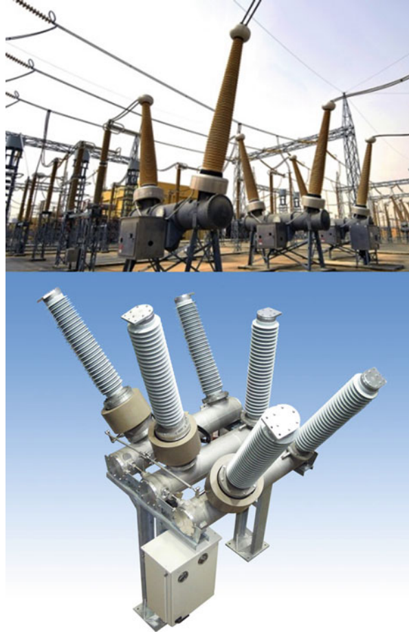
Fig. 12.4 (Top) Dead tank and (below) hybrid or mixed-technology switchgear
