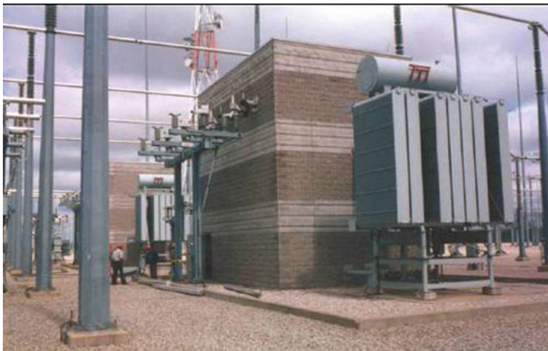
Fig. 11.33 Example of a sound enclosure (Canada)
