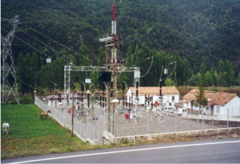
Fig. 11.46 The interior of the substation is visible through the chain-link fence
