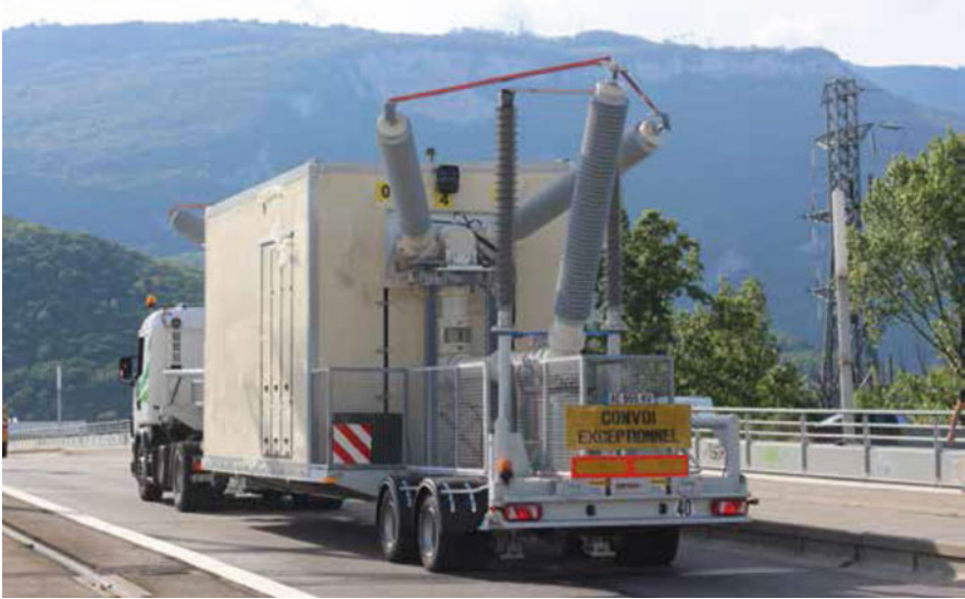
Fig. 6.3 Emergency mobile substation being transported to site
