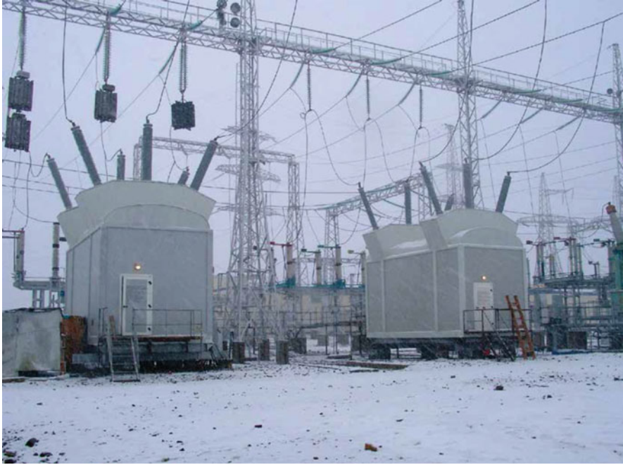
Fig. 6.5 Mobile substation being used to meet additional power demand
