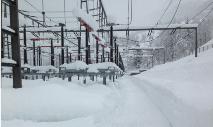
Fig. 12.23 Equipment and conductors coated with snow and ice
