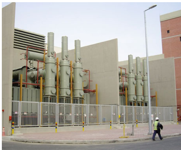
Fig. 18.8 GIS surge arrester with direct connection to the transformer via SF 6 insulated bus duct
