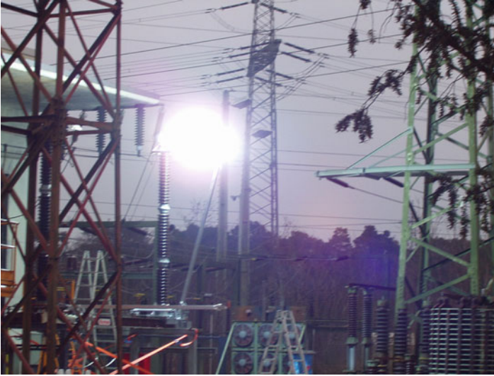
Fig. 5.9 Testing of a line end earth switch with whip contacts during 10 kV 400 A inductive breaking duty
