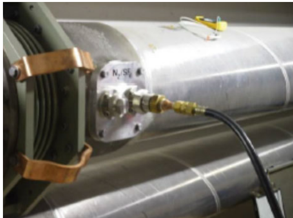
Fig. 27.33 Gas filling Dilo valve to vacuum connect gas handling device
