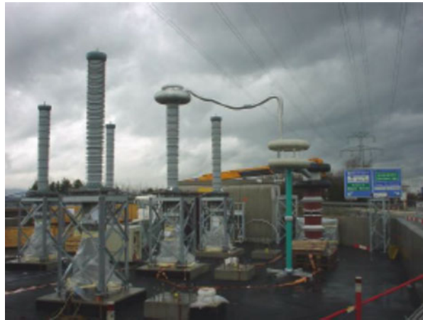
Fig. 27.35 On-site HV testing air insulated high-voltage resonance test setup connecting to the bushing
