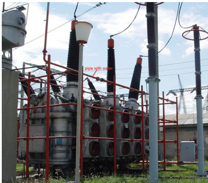
Fig. 11.34 Transformer fire suppression system using water in Romania
