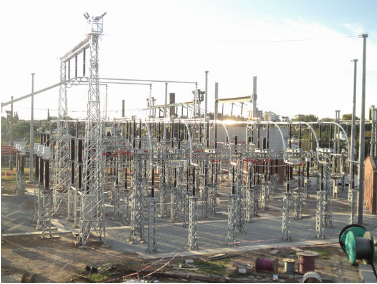
Fig. 26.5 Switchgear with only conventional components (CIGRE Brochure No. 390 2009)
