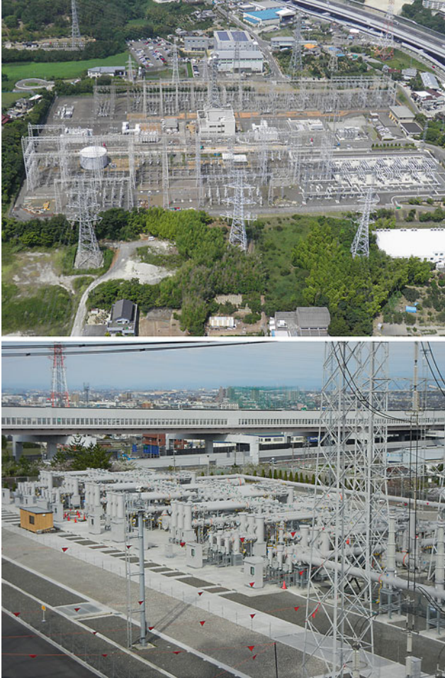
Fig. 15.4 Replacement of a former outdoor 14-bay-AIS substation (300 kV–50 kA) by a 14-bay-GIS substation. (300 kV–63 kA) (Chubu Electric Power Company, Higashi-Nagoya S/S)
