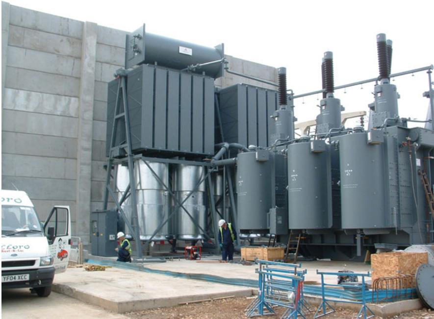
Fig. 5.13 Example of fire wall for transformer (during construction)
