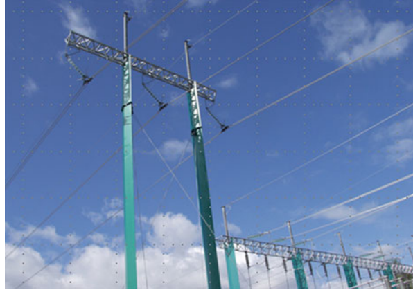
Fig. 42.2 The use of so-called landscape pylons in a 110 kV substation (Finland)
