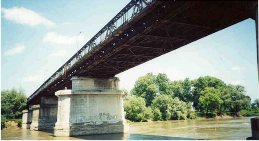
Fig. 6.30 A general view of the bridge across the Prut River in Chernivtsi
