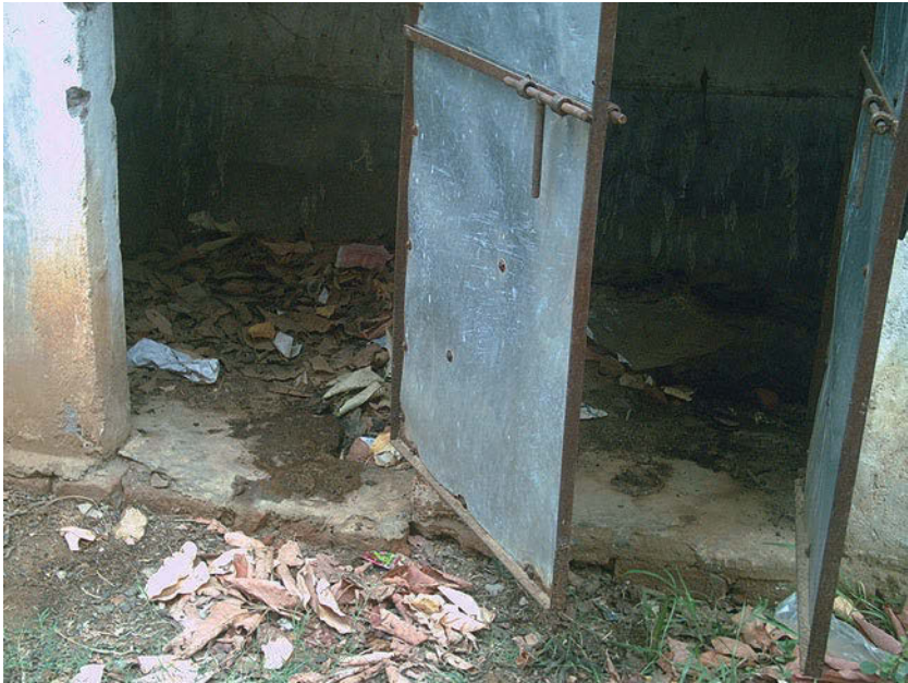
Photo 8.2 Dirty toilet facilities photographed by Parent 86
