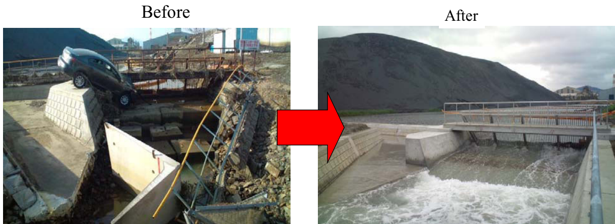
Figure 2 Photos of outlet port of discharge drainage
