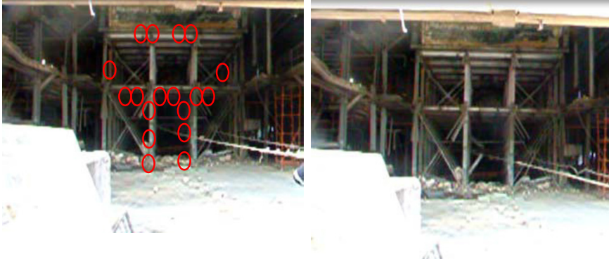
Fig. 2. (a) Furnace structure to be demolished. Red circles indicate where structure had been weakened; (b) Lateral load applied to structure to cause internal columns to pull out.
