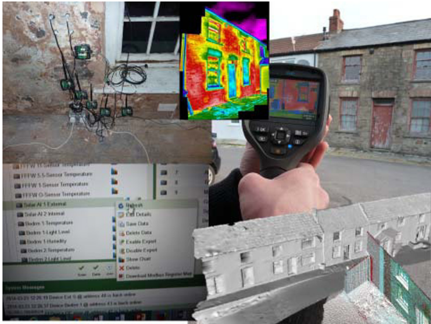
Fig. 1. A variety of forms of non-destructive measurement, and real-time data capture at the CADW cottage
