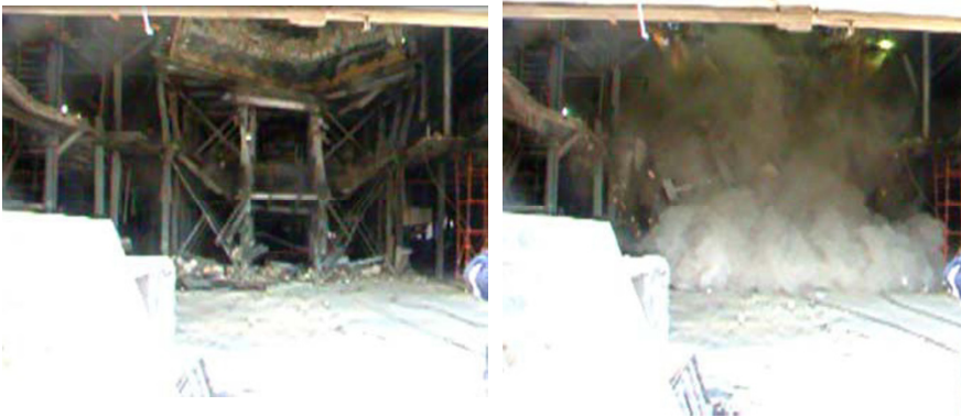
Fig. 3.(a) Structure in the process of collapsing after second line of columns removed;(b) Final pile of rubble which the demolition team could clear and recycle.
