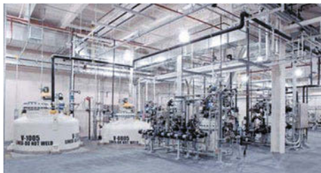
Figure 10 – Inside one of the solution treatment rooms in the “Pebbles Plant.”
