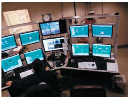
Figure 11 – The Materion “Pebbles Plant” that produces primary beryllium is controlled by several systems as the one shown.
