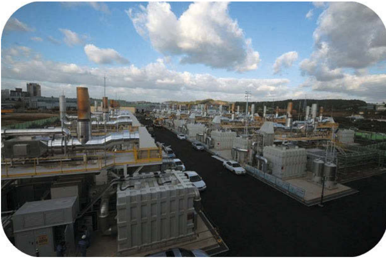
Figure 5. 59-MW, 5.2-acre fuel cell park (Photograph courtesy of FuelCell Energy)
