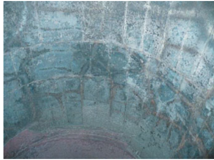
Figure 8: Hot Face of Lower Wall Bricks
