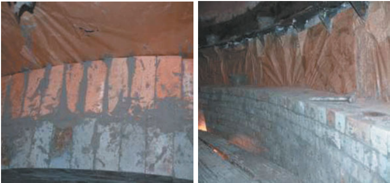
Figure1. Brick structure at CDQ's cooling section
