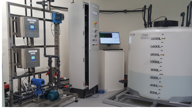
Fig. 6. Process P1 (raw water treatment) – SWaT testbed
