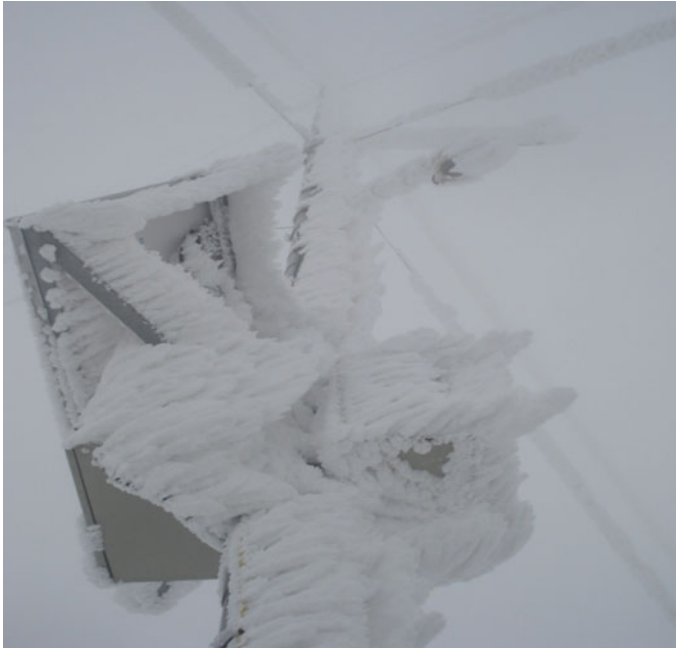
Fig. 4 Met-mast covered in snow and ice
