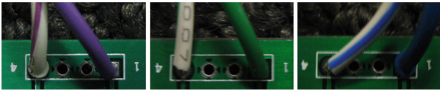
Fig. 10 Input wiring to Charlize boards
