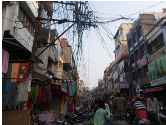
Fig. 8.2 Overhead web of power cables in Katra. Source Author
