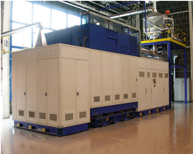
Fig. 1 Picture of the SOFC CHP-100 test site in TurboCare (Torino, Italy) Walpole and Myers (1993)
