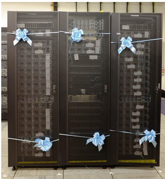
Fig. 1. The Panther system shortly after delivery to STFC Daresbury Laboratory; ribbons and bows courtesy of OCF plc.
