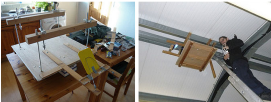
Fig. 20.3 Phase 1, (left) projector platform being constructed, note mirror cantilevered from the platform, and (right) installation at 5 m apex of Rural Centre roof
