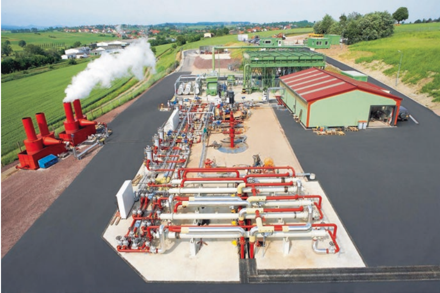
Fig. 5 Geothermal power plant at Soultz-sous-Forêts (©GEIE, 2009)
