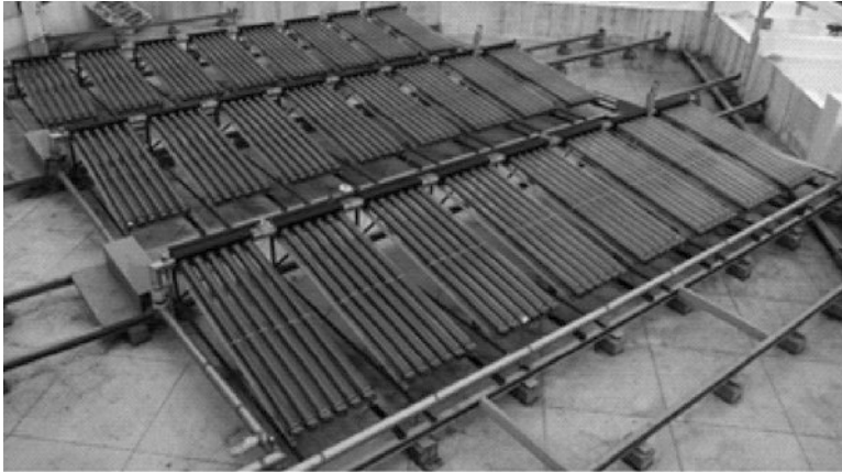
Fig. 1 Solar heating system used in the present study
