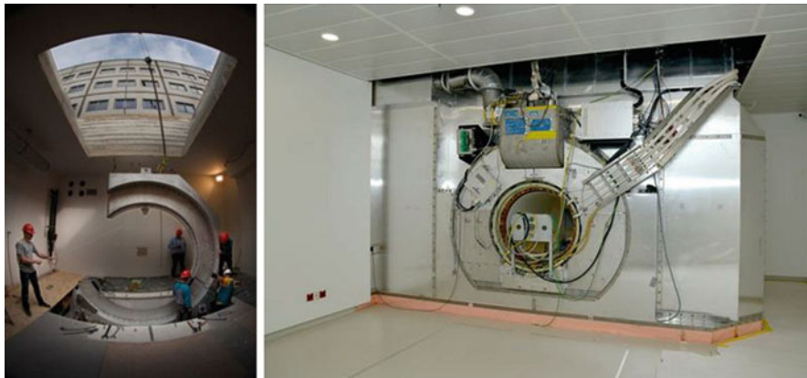
Fig. 5.15 UMC Utrecht installation of MRI/LINAC [70]
