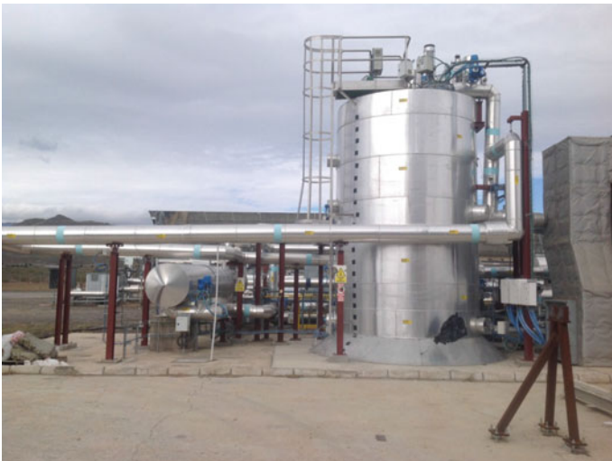
Fig. 3 Molten salt thermal energy storage facility at Plataforma Solar De Almeria (PSA), Tabernas Desert, Spain
