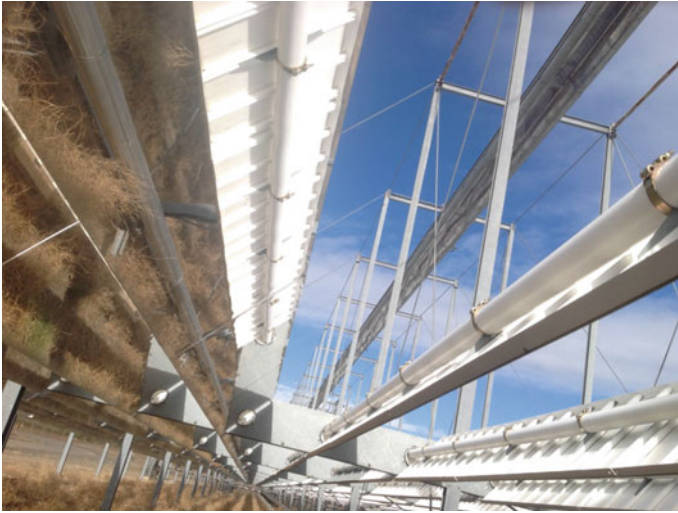
Fig. 2 Example of linear Fresnel CSP technology at Plataforma Solar De Almeria (PSA) facility, Tabernas Desert, Spain
